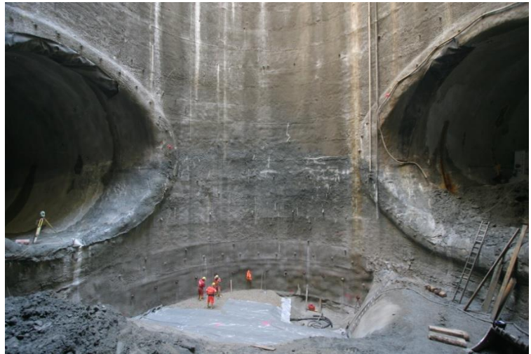
View of the cross shaft with NATM tunnel of the Koralm tunnel KAT2
